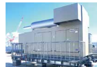
Emergency Generator (Ono Plant) [IBIDEN ENGINEERING CO., LTD.]
