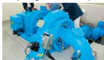
Low head hydro power system [IBIDEN Engineering Co., Ltd.]
