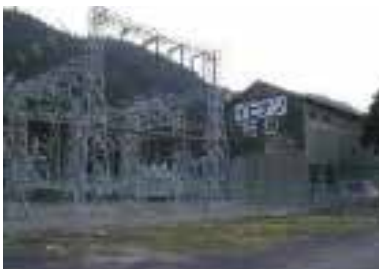
Hirose Power Plant (Updated in 2012) Power output: 8,900kW
