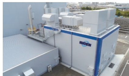
Cogeneration system (Ogaki Central Plant)
