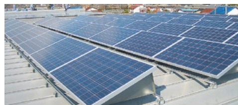
Solar power generation equipment
