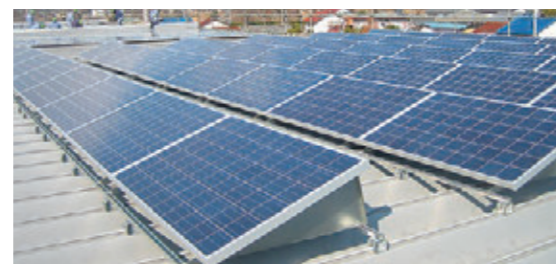
Solar power generation equipment
