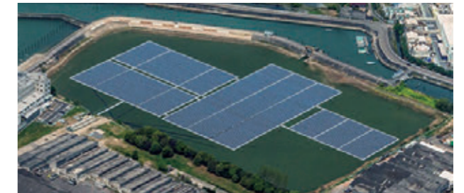
Water floating solar power generation plant (Kinuura Plant)
