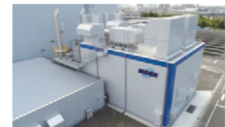
Cogeneration system (Ogaki Central Plant)
