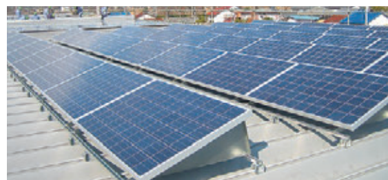
Solar power generation equipment
