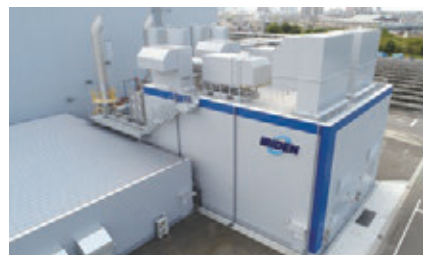
Cogeneration system (Ogaki Central Plant)
