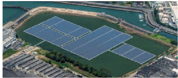
Water floating solar power generation plant (Kinuura Plant)
