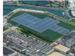
The Japan's largest water floating solar power generation
